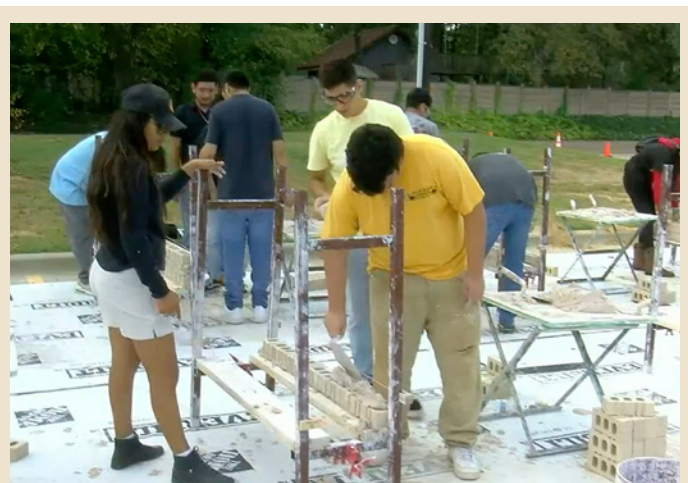
Students lay brick with supervision of local contractor Olvera Masonry Services, LLC.
